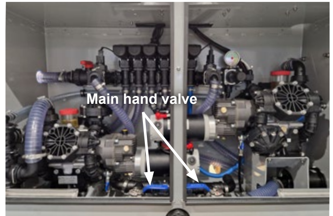
Main hand valve inside the stainless steel cabinet
